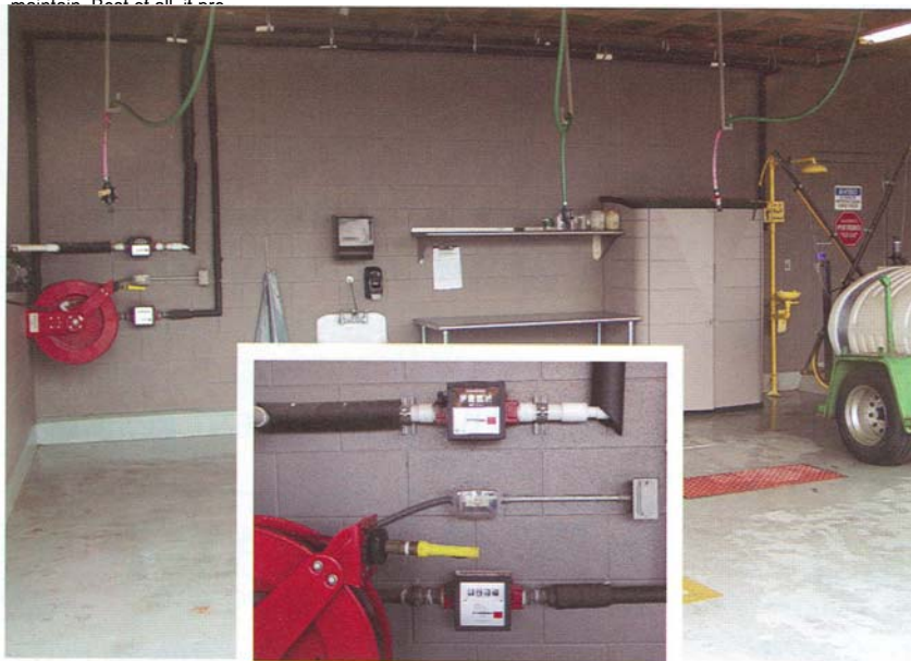
This is the main mix/load area. The concrete floor has a 36-mil chemical-resistant liner underneath and is sealed on top with chemical-resistant epoxy paint. The red grate covers the primary sump. A stainless steel mixing table, sink, eye wash and shower are some of the safety features. The recycled rinse water is stored in a 500 gallon tank to the left. Photo by Larry Livingston, CGCS.
